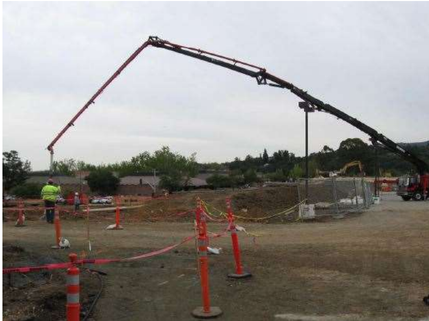
Figure 4. Cement truck pouring cement with a hydraulic arm (photograph by Peter Y. Chou).
