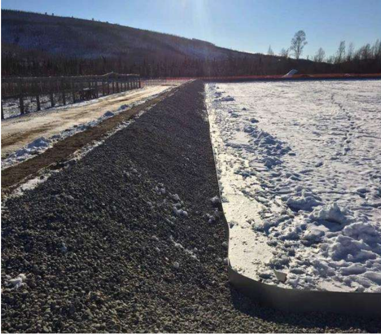
Figure B-8: Rock Armor and Flashing installation along southern side of Test Basin
