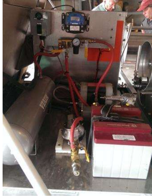
Figure 33: System Control Valves
