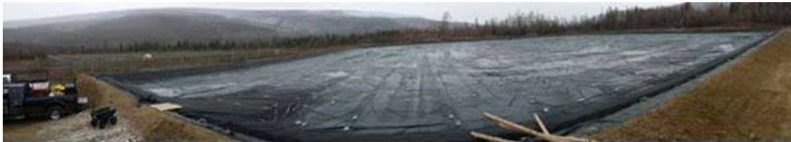
Figure E-4: Panoramic View of Finished Herder Test Basin with Liners and Geotextile Installed
