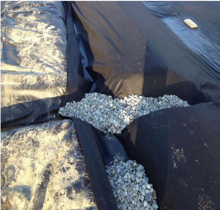
Figure B-5: Keyway with Liner and Geofabric and Rock Armor to Stabilize prior to backfill
